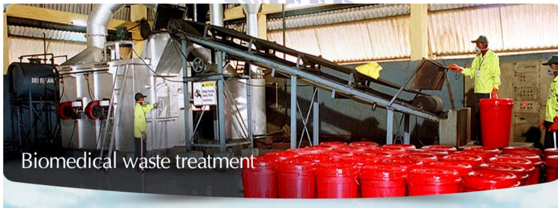
Figure - 8 Large Incineration Plant
